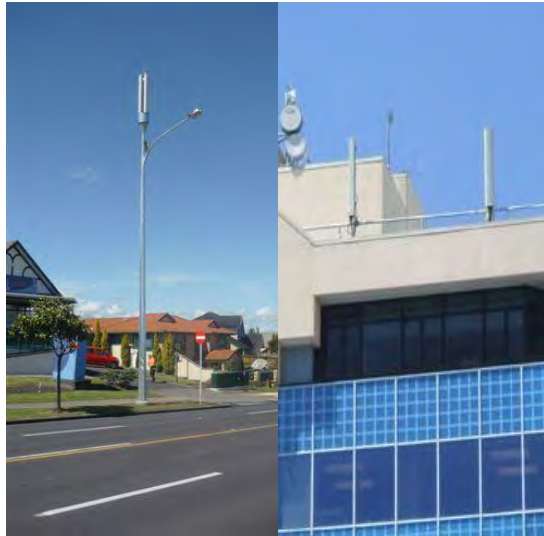
Figure 2: Examples of different mobile network antennas (in the photo on the right, the two structures are telecommunications antennas)
