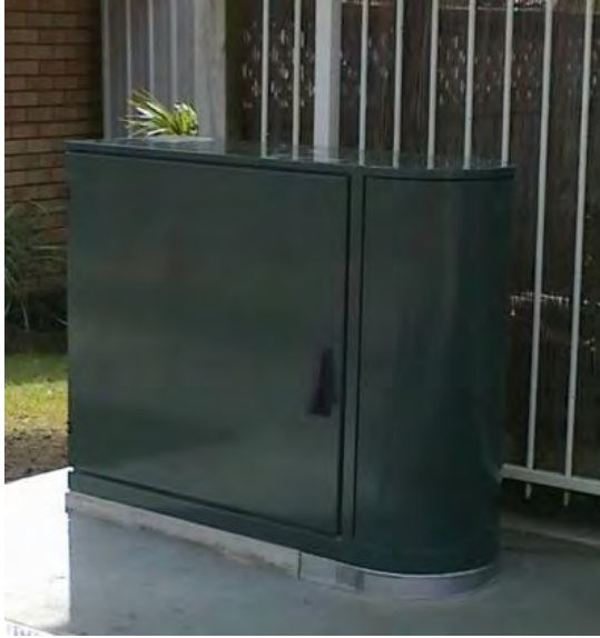
Figure A2.14: A fixed network street cabinet
