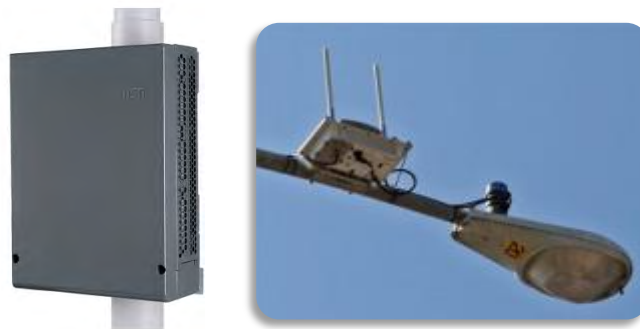
Figure 5: Example of a small-cell unit (left) and a pico-cell installed on top of a lamp-post (right)
