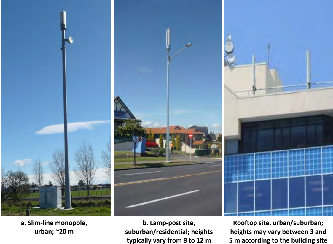
Figure A2.10: Examples of different installed antennas
