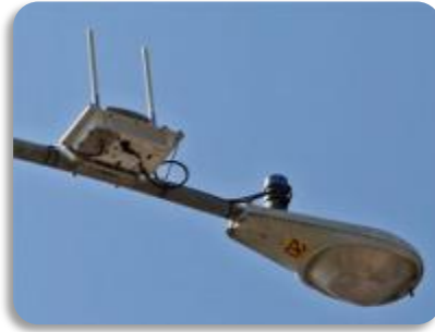
Figure A2.12: A pico-cell installed on top of a lamp-post
